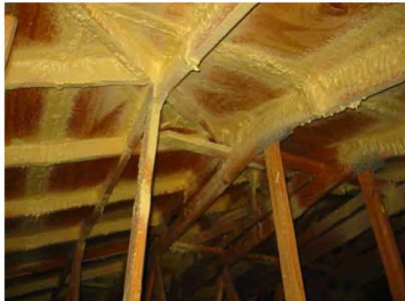
Figure 1. Closed-cell polyurethane foam adhesive applied to the underside of the roof sheathing at the joints between the sheathing panels and along all intersections between roof sheathing and all roof framing members.
